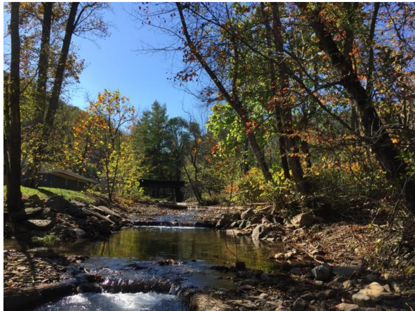
Cross vanes installed along Wyckoff Run. Cross vanes deflect high flows away from the stream banks and help form deeper pools
